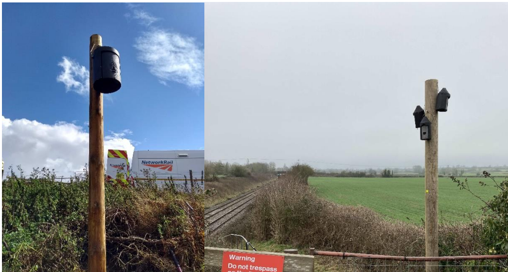
Figure 5 Photos of bat boxes installed as mitigation for vegetation management works in Western (Photo credit: Morgan Sindall)
