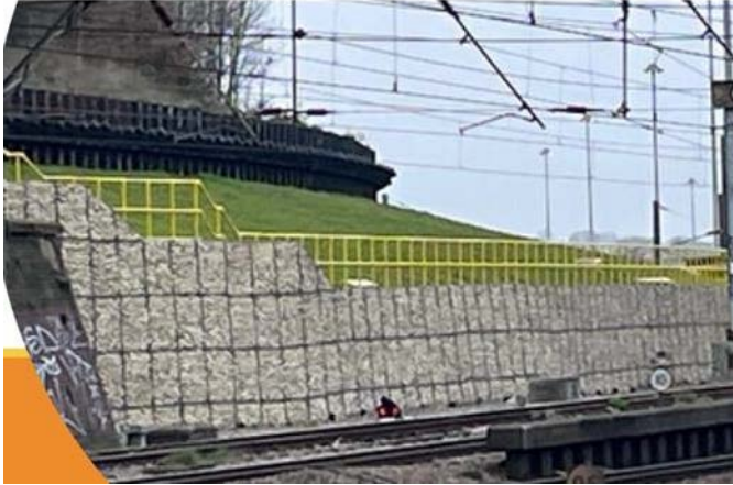
Figure 5.2: Original design for bank stabilisation and retaining wall prior to engaging with the London Wildlife Trust.
