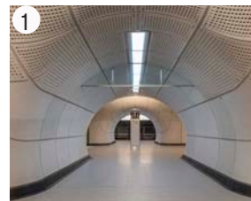
Image 4.49: Ceiling mounted luminaires
