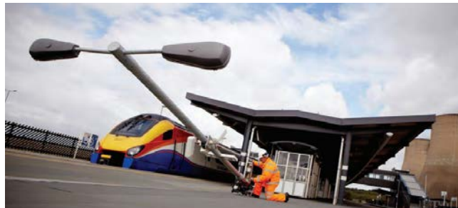
Image 7.6: Base-hinged lighting columns provide ease of access at ground level.
