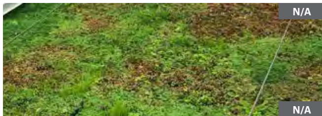
Green Roof - Extensive
