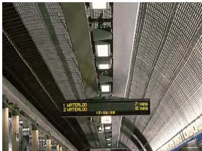
Image 3.6 London Bridge Underground - Integrated containment
