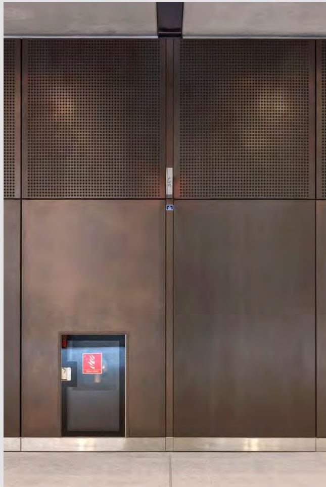
Image C.3 Prefabricated bronze cladding units line the ticket hall with integrated acoustic treatment behind their perforations
