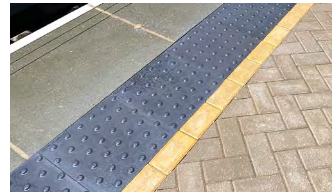
Image 1.30 Platform edge tactile paving
