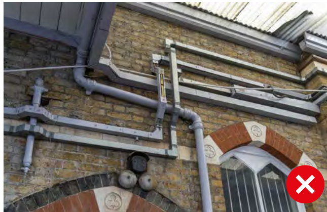
Image 3.5 Example of ad-hoc and poorly managed / coordinated containment.
