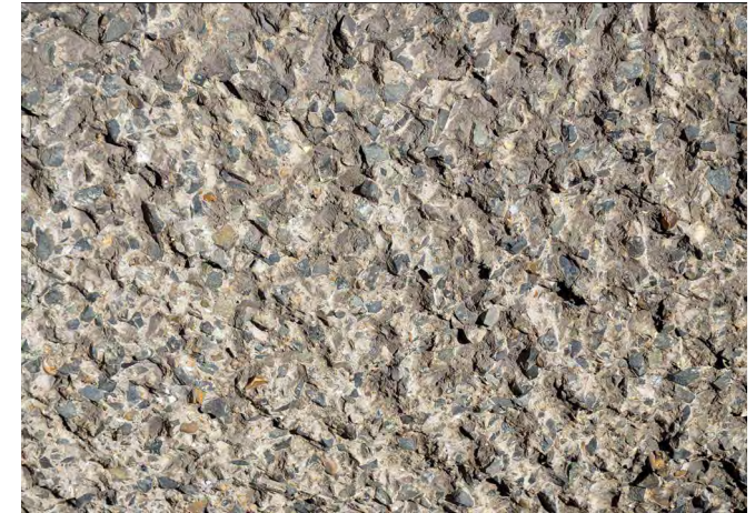
Image 2.45 Tooled concrete finish by pick and bush-hammering to expose the aggregate at the Barbican, London
