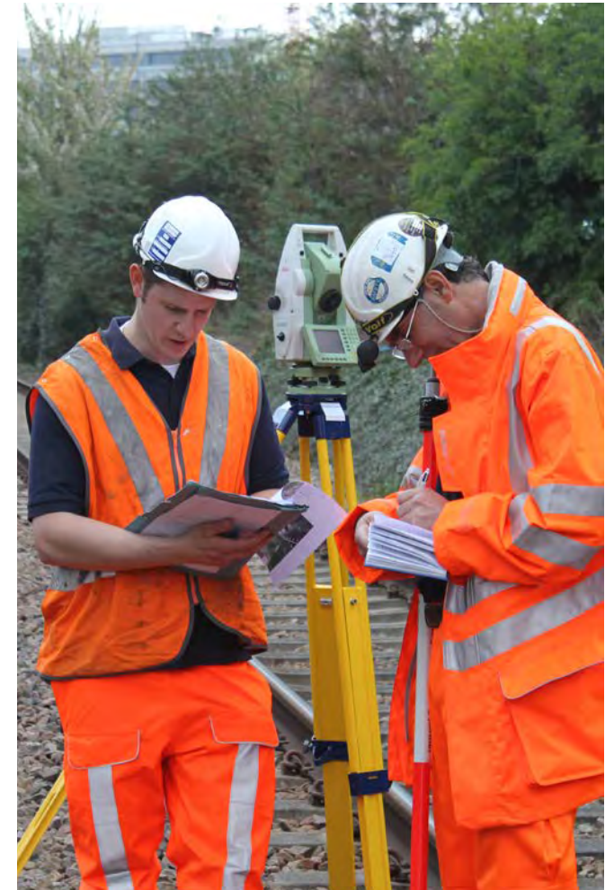
Image 4.1 Precise survey information helps to maintain the safety and integrity of railway infrastructure
