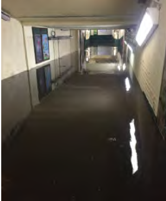
Figure 27 Flooding at Carnforth station subway
