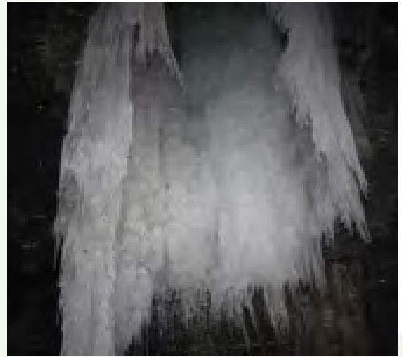
Figure 23 Ice build-up – Birkett Tunnel
