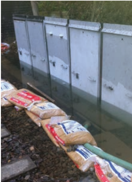
Above: Flooded signalling equipment Collaborative working with First Great Western during extreme weather. In early 2014, trains travelling into and out of Paddington faced a 20 per cent reduced service to normal due to signalling equipment at Maidenhead being under several feet of flood water. We worked innovatively with First Great Western, including introducing a temporary signalling system and a revised timetable, to bring service in excess of 75 per cent normal.
